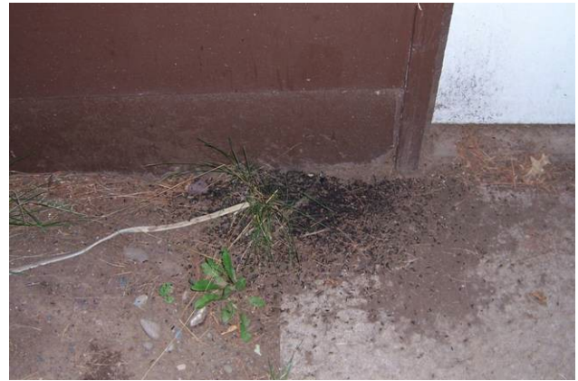
Bat guano in front of garage
