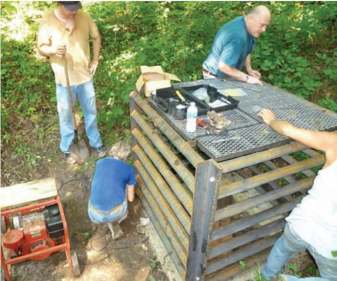
L to R: David Redell, Hans Verick, Tom Kesselhon, and Gary Emerson work to install a bat-friendly gate over the small entrance to the Star Valley Cave.
